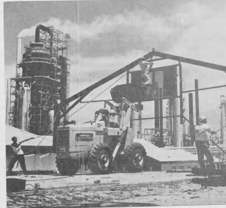
QUICK WORK was made of dismantling the old Zone 2 building's steel frame. Steel cables were merely secured to the beams and to a powerful tractor.
